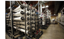
Photo: Reverse Osmosis Unit
