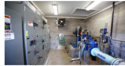
Photo: Well Pump House
