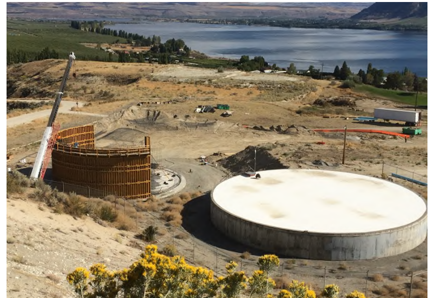
City of Brewster Water Reservoirs
